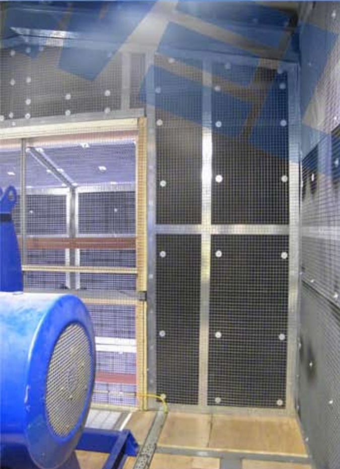
Insulated Fan house complete with insulated air inlet
